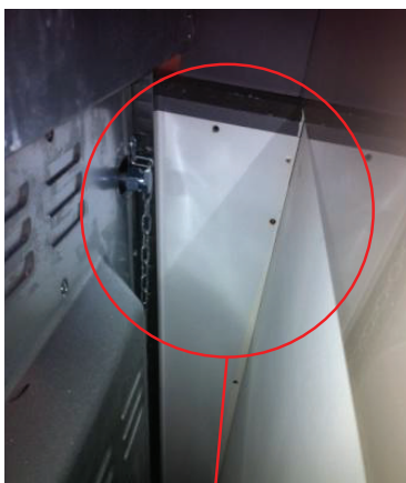
Left side of the oven: Chain not attached.
